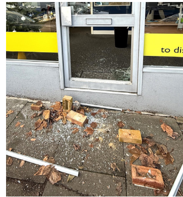
Criminal damage: The Tax Assist office
