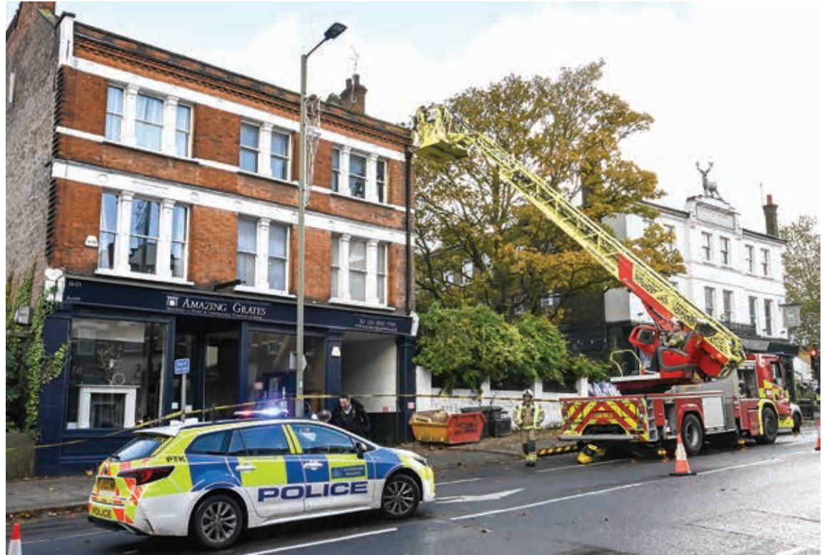
Long drop: Fire crews make safe the broken masonry and brickwork above the Amazing Grates shop. Photo Mike Coles
