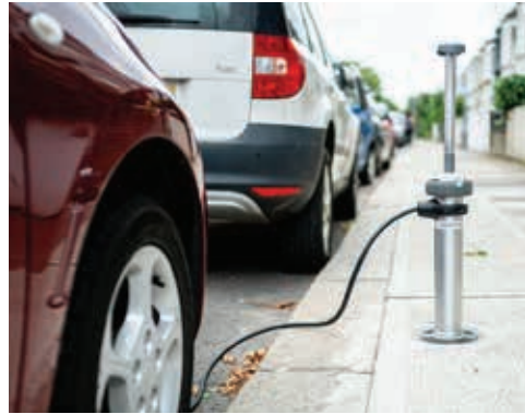
Pavement power: One of the new street chargers in action
