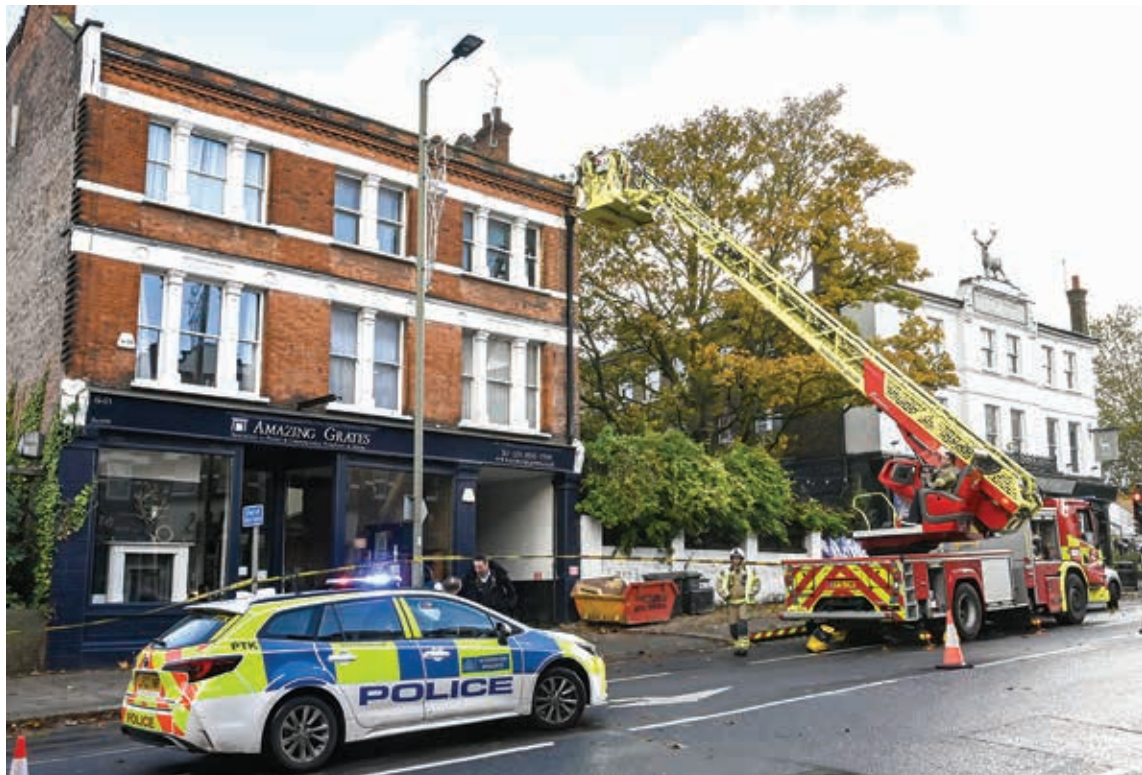
Long drop: Fire crews make safe the broken masonry and brickwork above the Amazing Grates shop.
