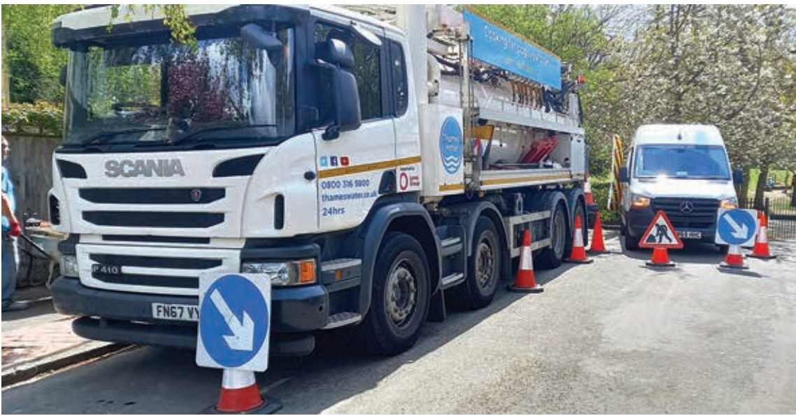
Going underground: A Thames Water tanker in place for the drainage inspection at Cherry Tree Wood.
