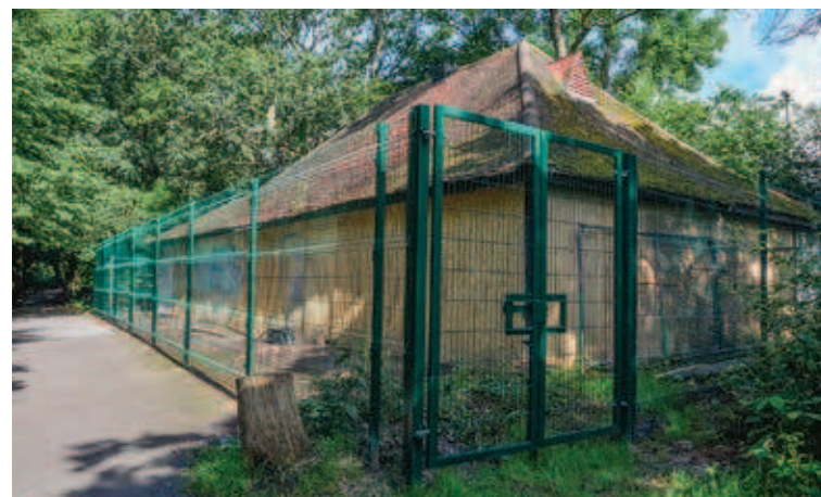
The current state of the Cherry Tree Wood pavilion. Photo Mike Coles
