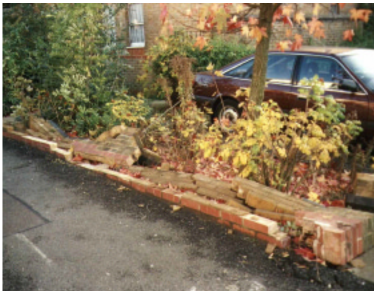
Damaged walls in King Street. Photo by John Dearing
